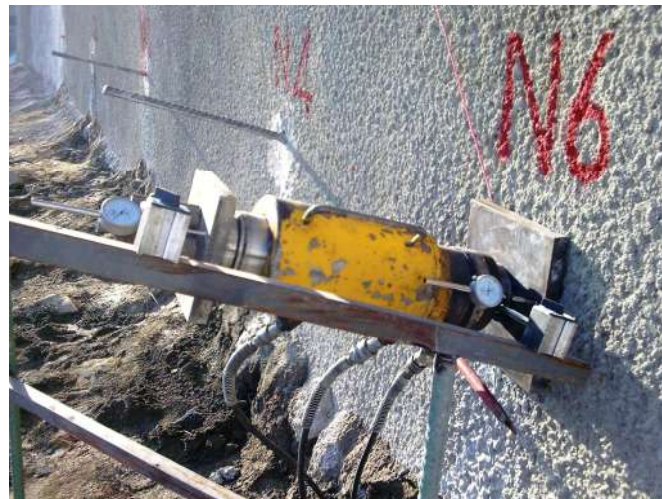
Figure 3. Photo of the Test Apparatus during the test.
